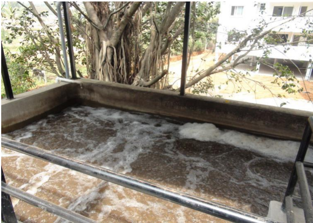
Water treatment in Aeration Tank
