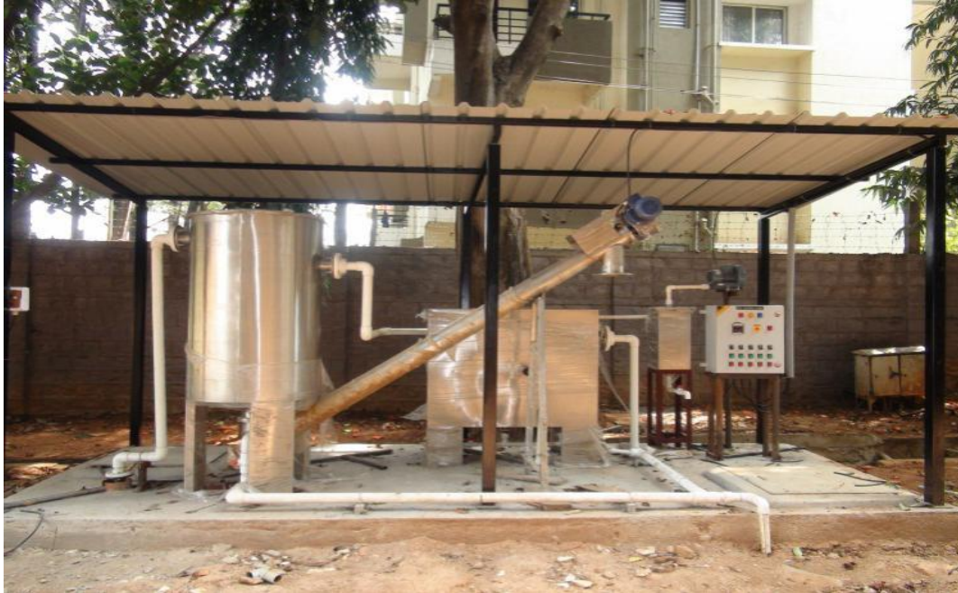
Separation of oil & Grease from waste water
